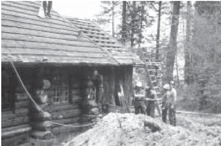
Lake Tahoe Basin Management Unit: Nevada Air National Guard, one of many site preservation partners, rehabilitating one of the buildings at Tallac Historic Site.
