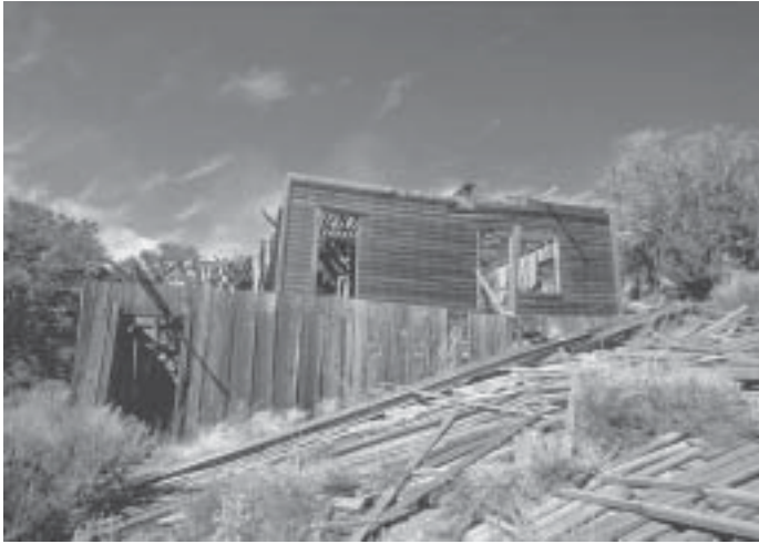
Figure 2: Dilapidated tender's cabin, 1998.
