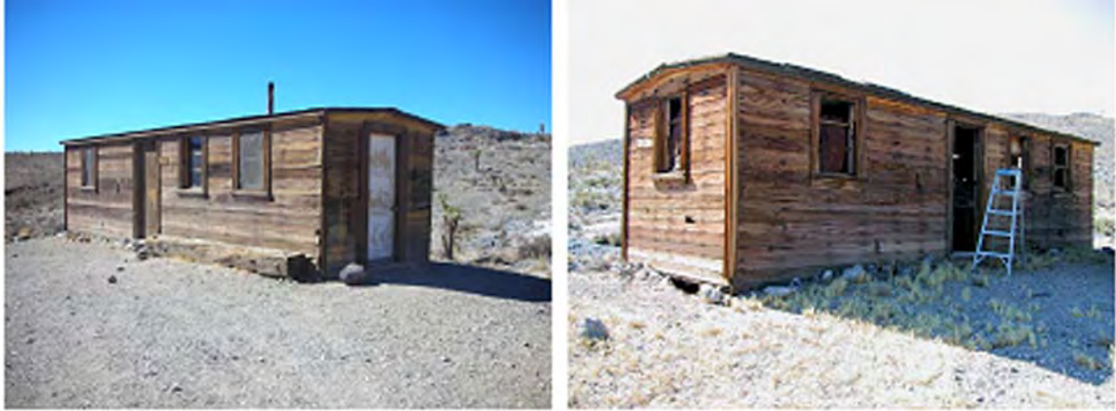
Figure 7. (left) Boxcar Cabin after stabilization, view toward southeast; (right) prior to stabilization work in 2003, view toward southwest. (Photograph: Friends of Boxcar Cabin)
