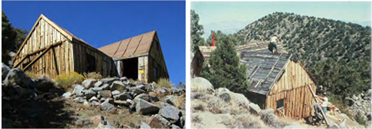
Figure 1. (left) Beveridge Cabin in 2006, view northwest; (right) undergoing stabilization (ca. 1990), view southeast.
