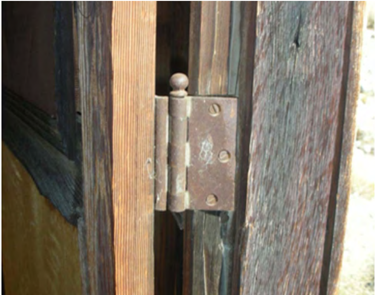
Figure 6. Door repair showing planed surface on door edge, replacement panel (at left) and reuse of original ball top hinge.
